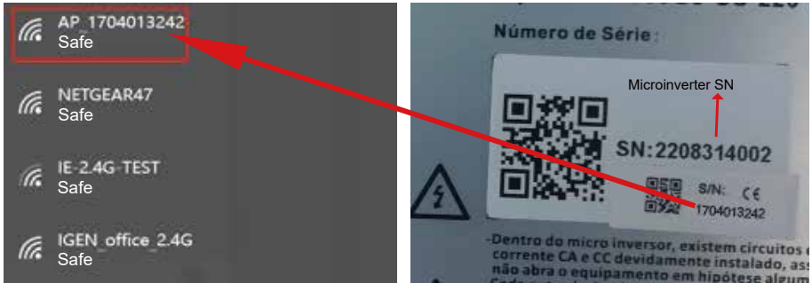
Microinverter SN: 2208314002 Built-in datalogger :1704013242
